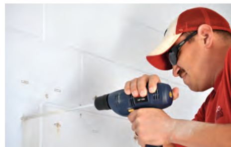
Sean Stull of St. Francis of Assisi Council 10994 at Joint Base McGuire-Dix-Lakehurst in Wrightstown, N.J., drills holes for wall anchors while mounting a flat-screen TV at the base's chapel complex. Long underutilized, the facility needed to be made ready for a new influx of religious education students. In addition to painting and carpeting the chapel and its 22 classrooms, Knights also installed televisions, DVD players, whiteboards and corkboards in each room.
